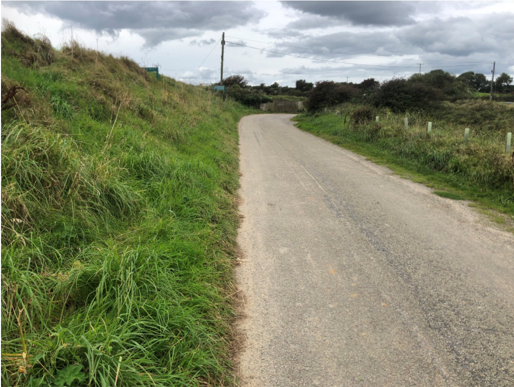
Photograph No.3: View of Existing Roadway taken in or around CH1100 looking west.
