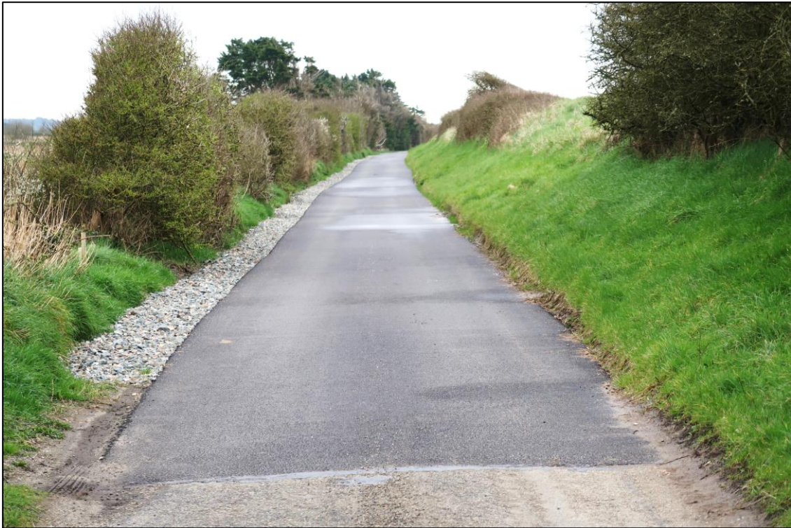
Plate 7. Emergency repair works on a pot-holed section of the road that was breaking up, with stone filling (left) to attenuate surface rainwater runoff. Note that from this point on the road is screened from the sloblands (left) by vegetation.
